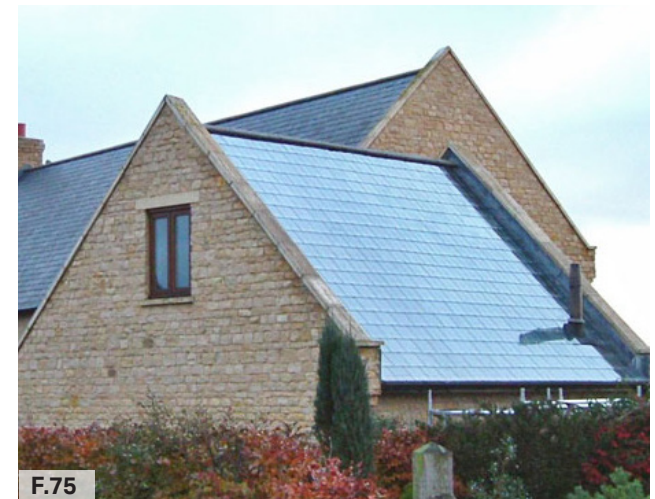
Figure 75: Positive example of integrating solar panels at the design stage.
